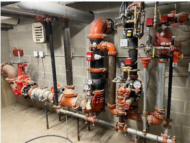
Sprinkler room in a mixed-use occupancy
